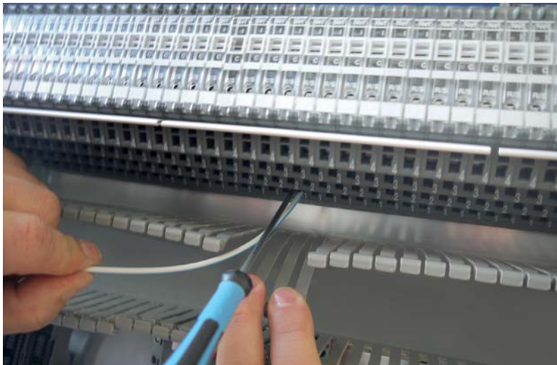
By comparison: Back panel - obstructed by wiring ducts
