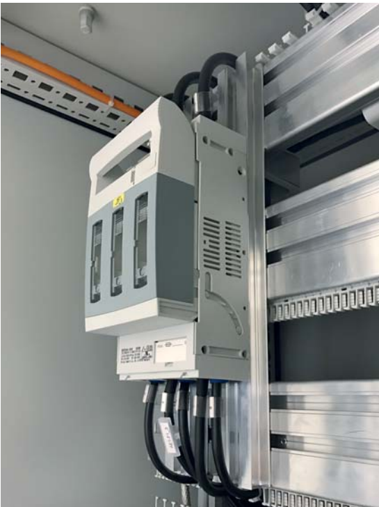
Fig. 1: Master switch to RG 035.
